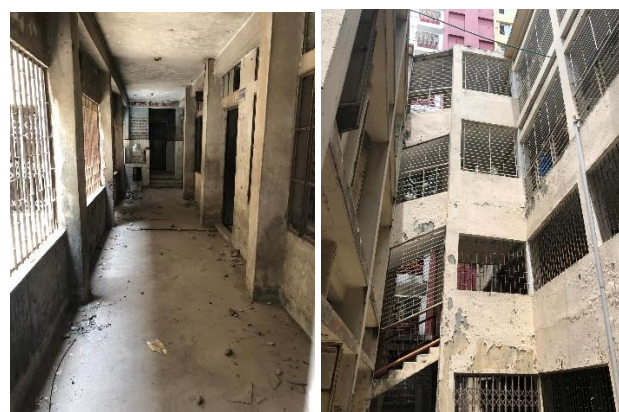
Figure 10: Building and settling condition
