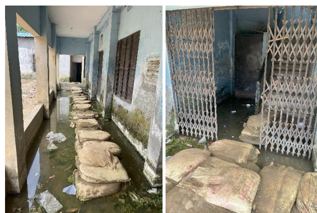
Figure 4: Waterlogging condition at the entrance
