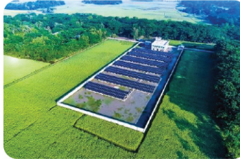
Solar Mini-Grid Project at Jamalpur
