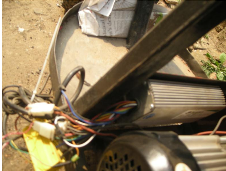
Figure 5.5.8 : a. Control Unit
