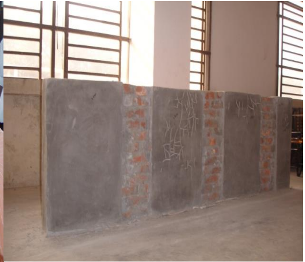
Figure 6: Crack formation on plastered surface
