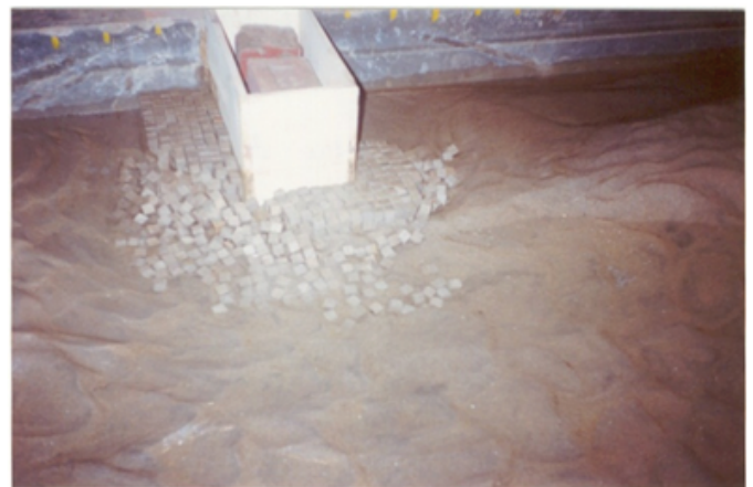
Fig 21. State of apron material on the scour hole
