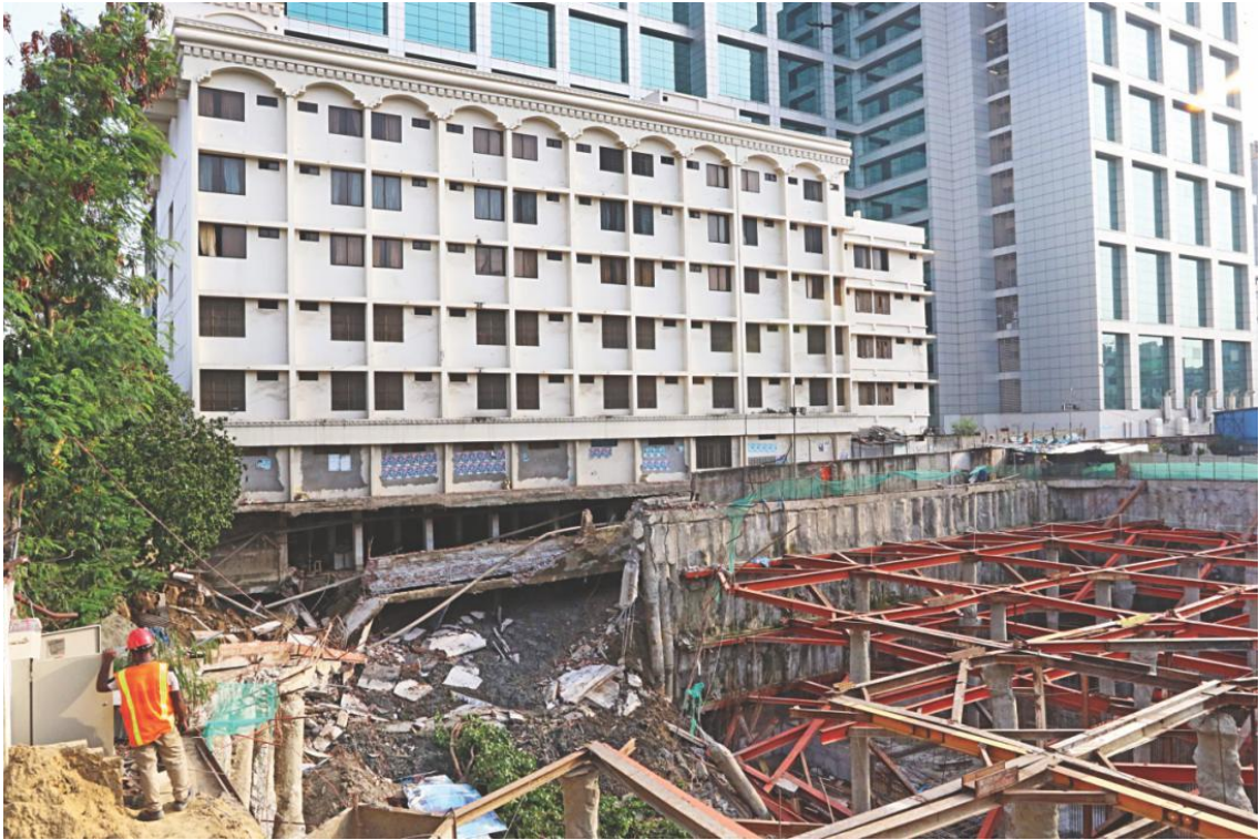
(a) A six-storey building in capital Dhaka's Karwan Bazar has been evacuated after a street beside it suffered sudden subsidence.
