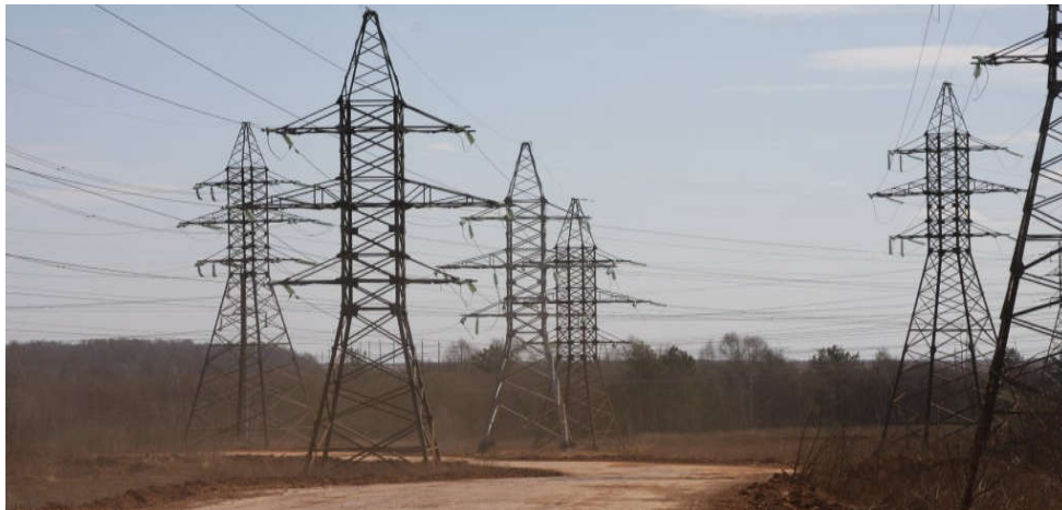
Fig- 4.1: Overhead Line
