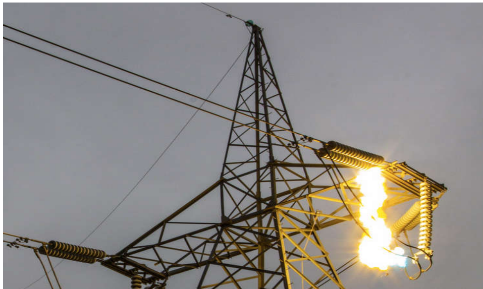
Fig-5.1: Short circuit fault in a tower
