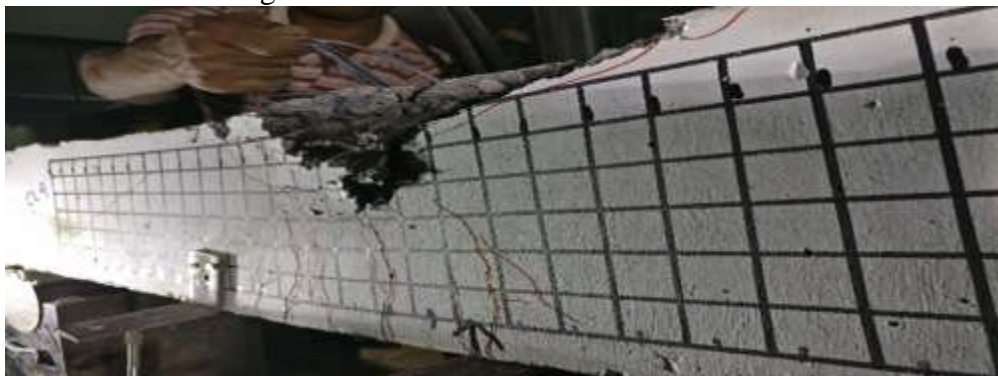
Fig 4. 20 : Crack Pattern for beam MSH-1
