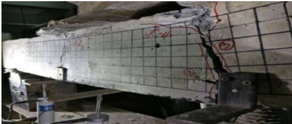
Fig 4. 1: Crack Pattern for beam SSL-1
