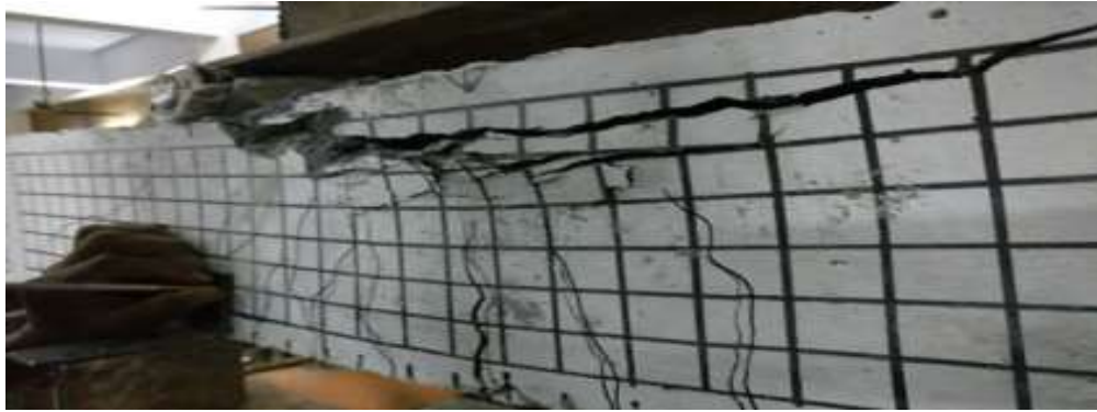
Fig 4. 21: Crack Pattern for beam MSH-2
