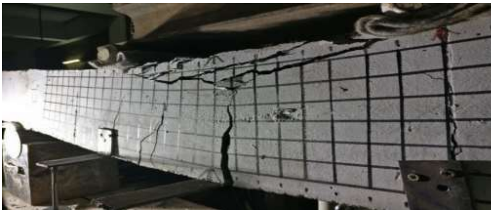
Fig 4. 4 : Crack Pattern for beam MSL-2
