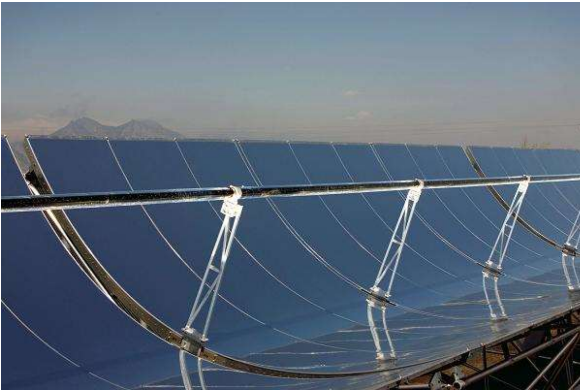
Figure 2.3.3: Parabolic Trough Solar Collector
