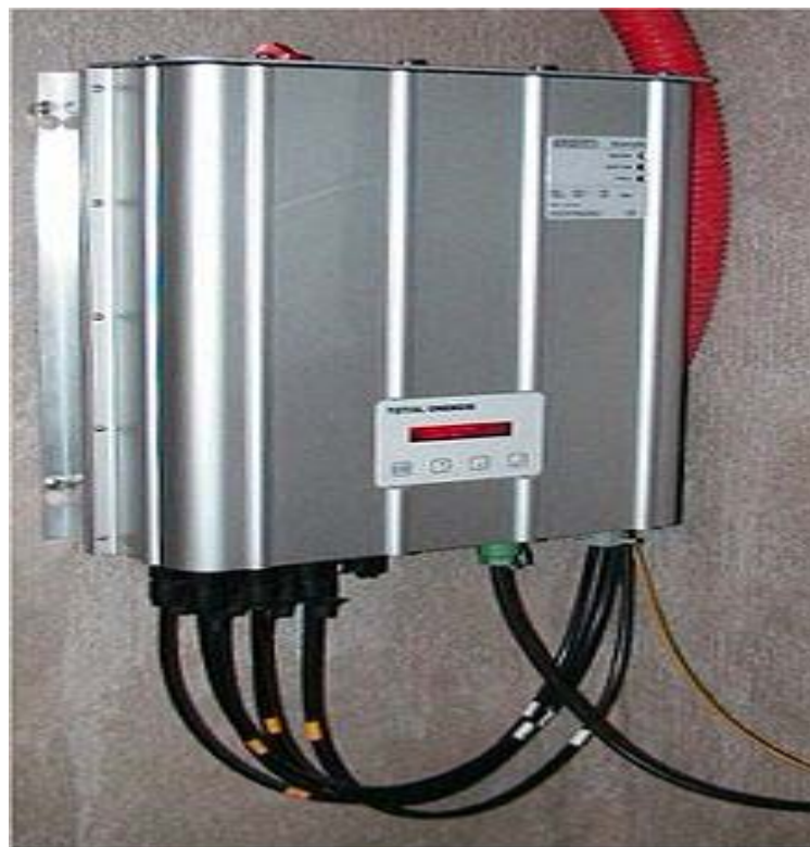
Fig: 3-11. Inverter for grid connected PV
