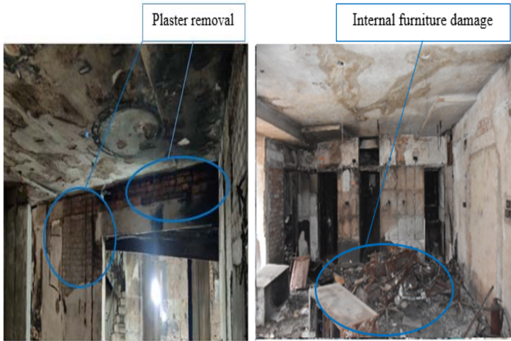
c) Plaster removal in front of the stair on the 8 th Floor (Grid-B,C/3,4)
