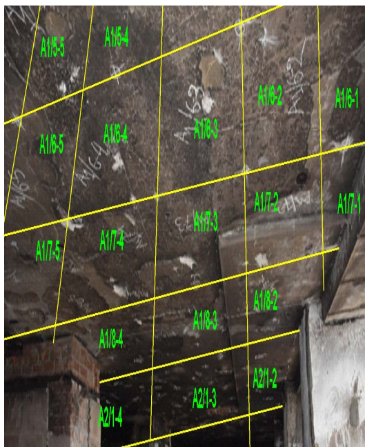
a) 900 mm X 900 mm subdivision at the 7 th floor roof slab (Grid-A, B/1,2)
