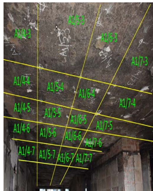
b) 900 mm X 900 mm subdivision at 8 th floor roof slab (Grid-1,2/A, B,C)
